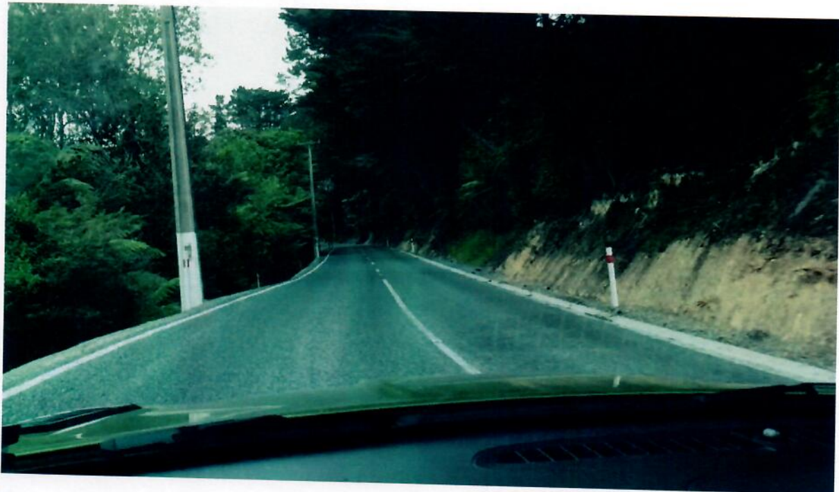
Photograph 12: No Edge Marker Posts (ch.940)
