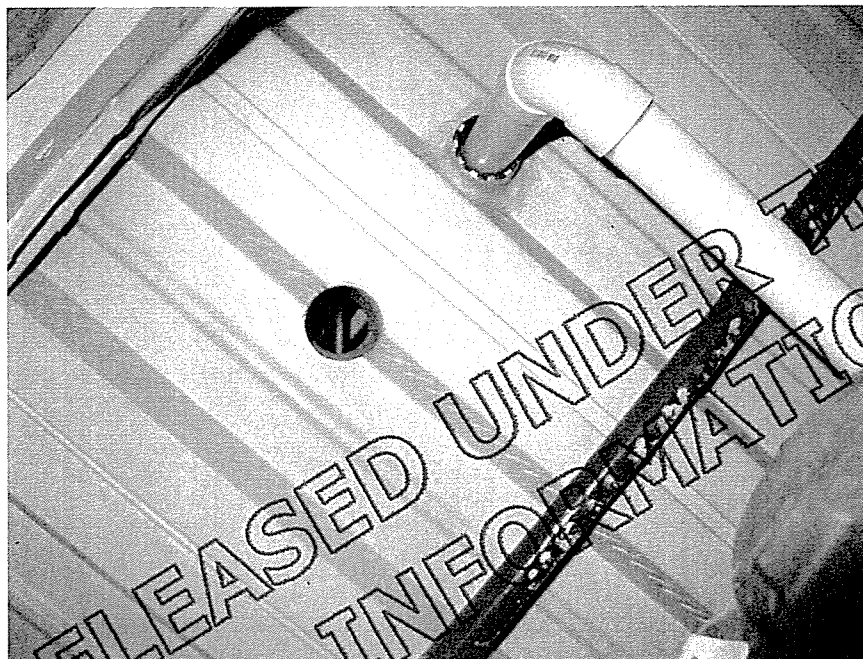
Figure 5.1.4 – Hole in fire-rated floor
