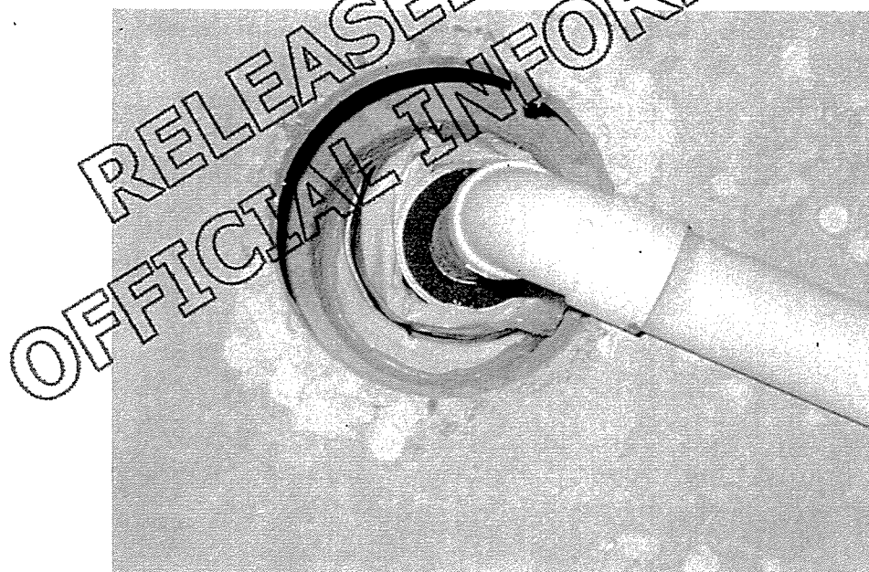
Figure 5.1.1 – Oversize hole for shower waste pipe
