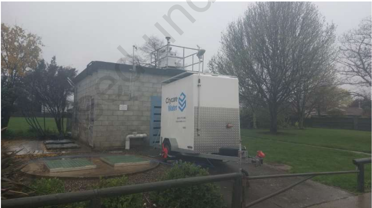
Figure 6-2 DTSx3000 unit in trailer at Goodman Park Pump Station
