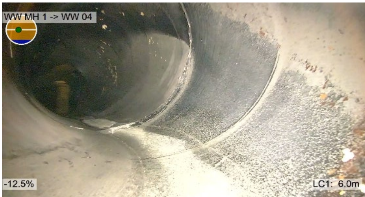
Figure 3-20: OD1371 CLS Effluent pipe View downstream of 35 degree horizontal bend. Spiral pattern and staining or erosion of polyurethane lining evident for full circumference downstream of bend.
