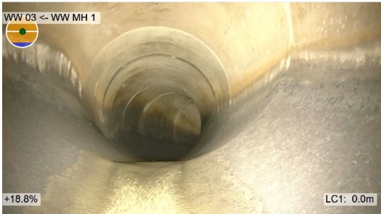
Figure 3-17: OD1420 Effluent pipe CCTV footage looking in upstream direction from the bypass junction tee towards HB1. Shows steep downward bend immediately upstream of the bypass junction which is not recorded in the As Builts. Grade around HB1 appears consistent.
