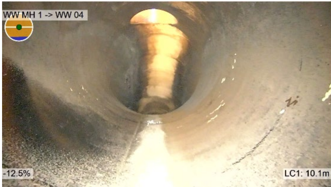
Figure 3-21: OD1371 CLS Effluent pipe View looking downwards towards air valve tee. Erosion and staining extends high up pipe to soffit level as far as the air valve tee and 15 degree downward bend. Coarser surface roughness in invert is observed here.
