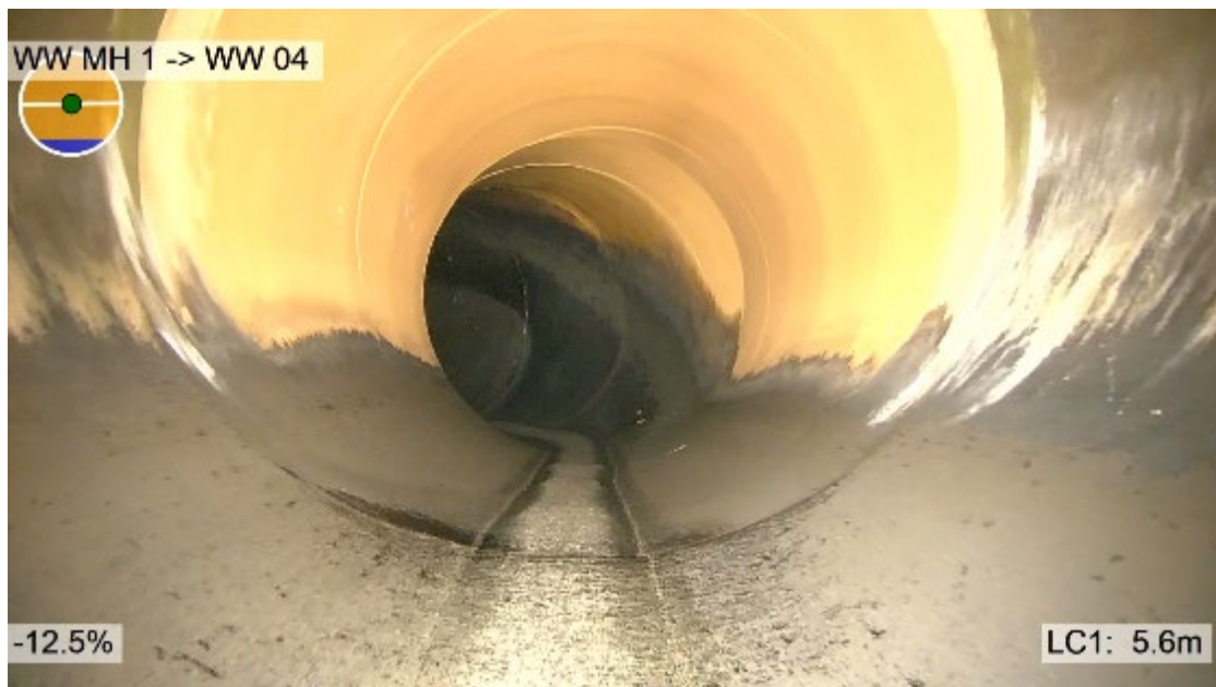
Figure 3-18: OD1371 Effluent pipe upstream of 35 degree horizontal bend. Shows transition to section with additional polyurethane lining and erosion of polyurethane lining in invert. Inaccuracy in CCTV distance noted.
