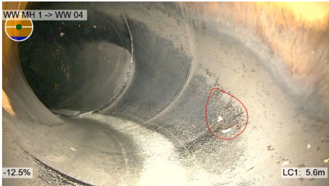
Figure 319: OD1371 CLS Effluent pipe at 35 degree horizontal bend. Erosion of polyurethane lining is evident up the wall on outside of bend. Potential pitting of cement mortar lining circled in red (camera does not zoom at this location).
