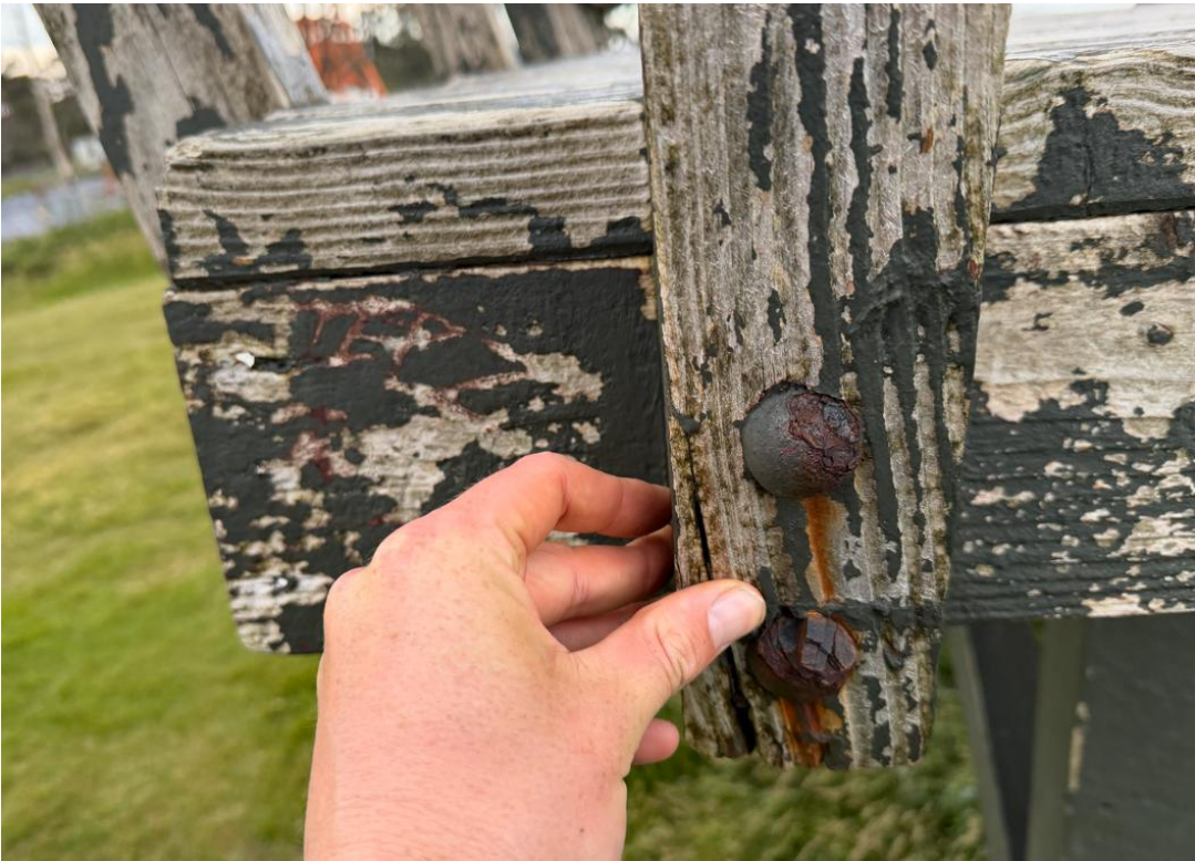
Figure 3 Corrosion and inadequate spacing at barrier post bolts - Photo taken by Frame Group on 5 Dec 2025.
