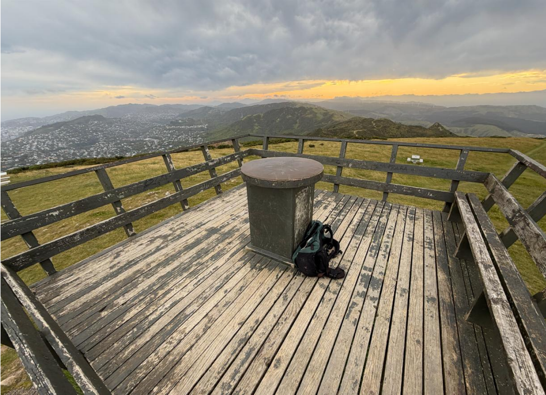
Figure 2 Mt Kaukau Lookout Platform (Asset #20006501) - Photo taken by Frame Group on 5 Dec 2025.
