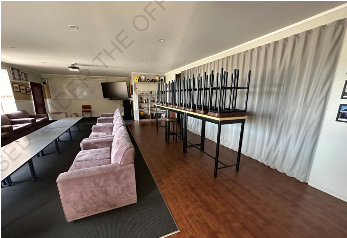
Large void behind curtain in social room to appliance bay wall.
