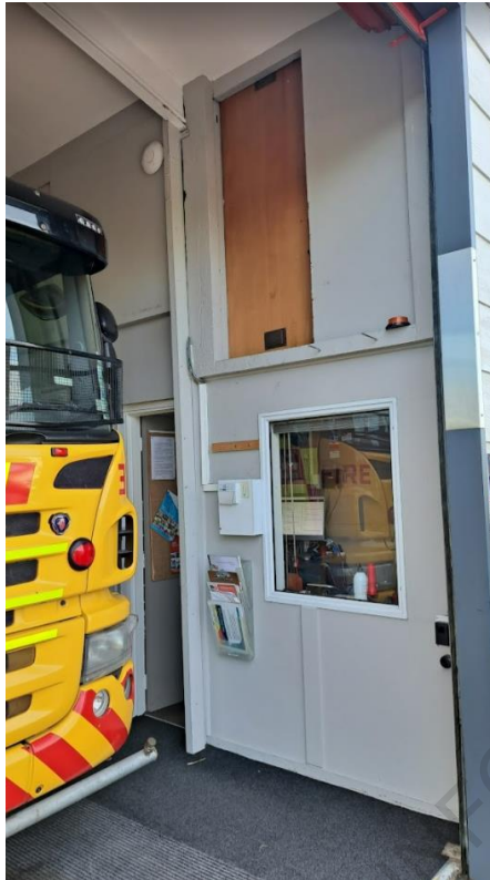
Penetrations in appliance bay side bracing walls. Steel roof rafter can be seen, boxed out in white plasterboard. The post can also be seen on the left high-level door.
