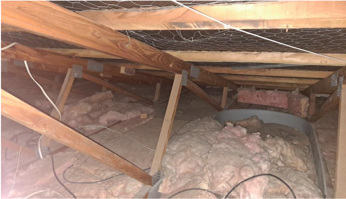
Lean-to roof truss system
