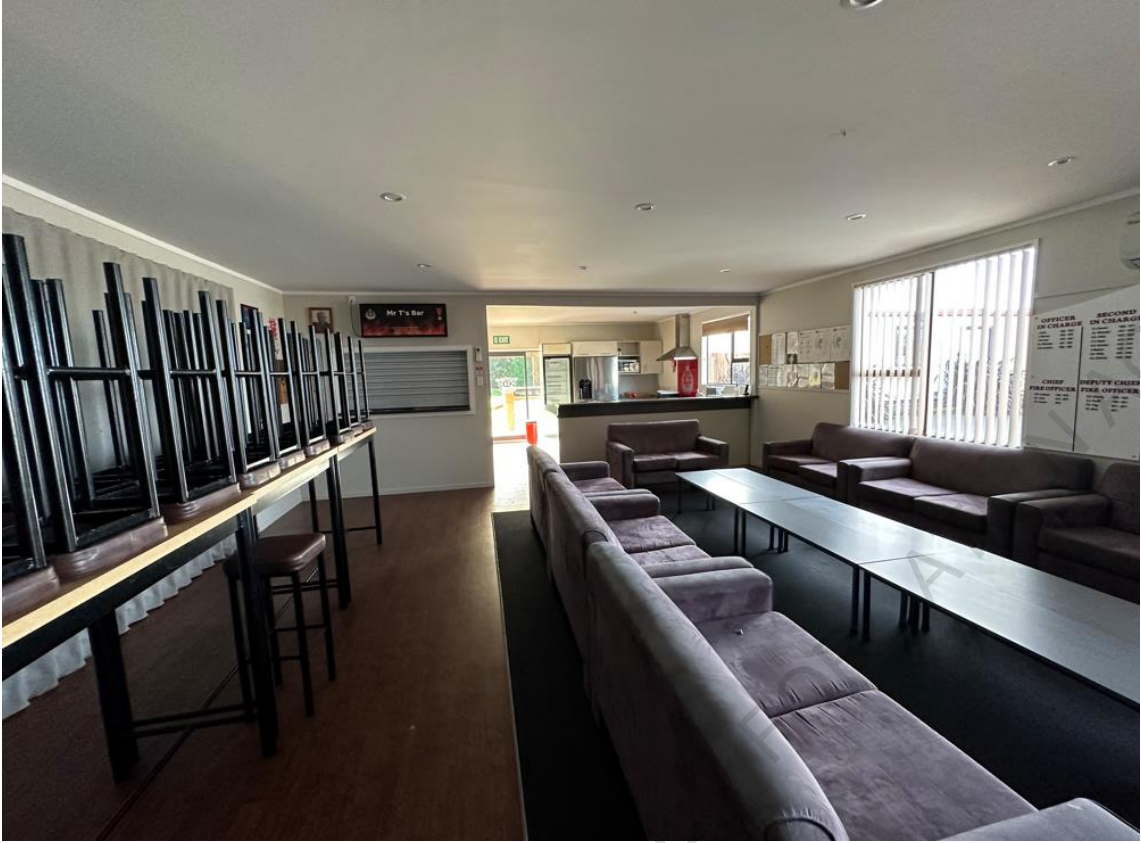
Large voids in kitchen area wall.
