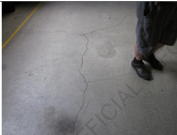
Cracking in floor slab
