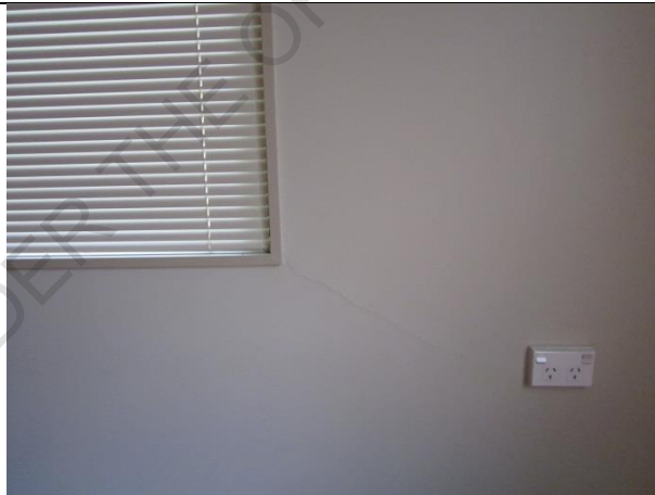
Internal Elevation – cracking in plasterboard beside window on first floor
