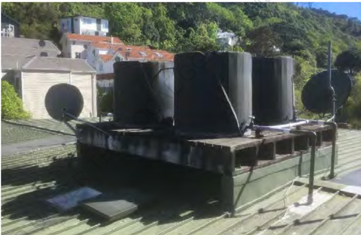
The tanks at roof level are supported on a timber platform with no apparent seismic system.
