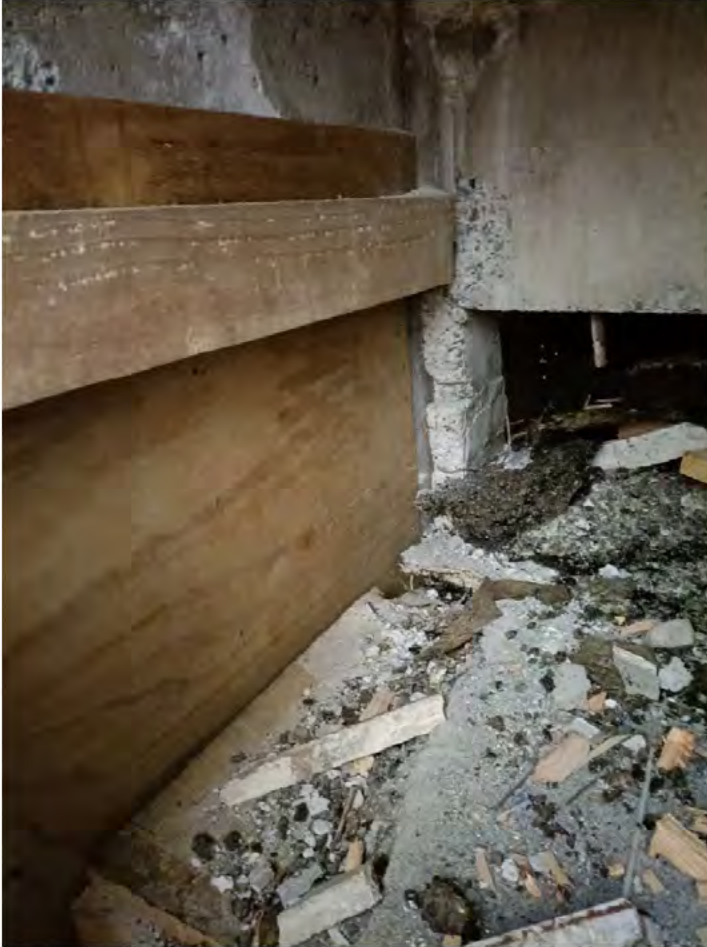
Interior of plywood wall on Glenmore Street elevation and cast-in steel beam
