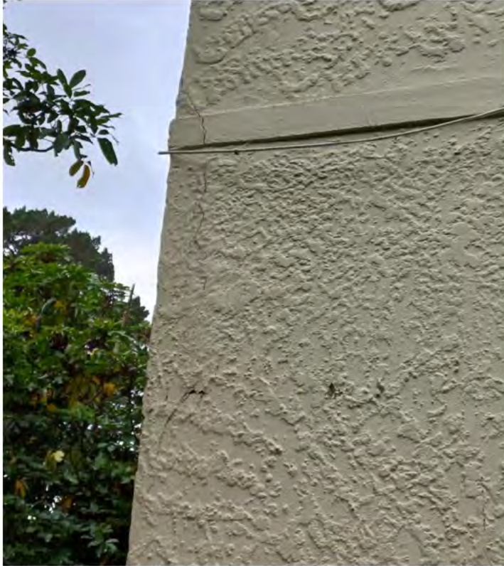
Cracking at Glenmore/Driveway Corner (Grid F/5 intersection)
