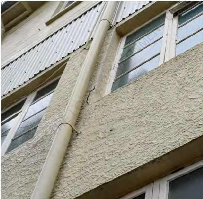
Cracking on Grid 1 pier.
