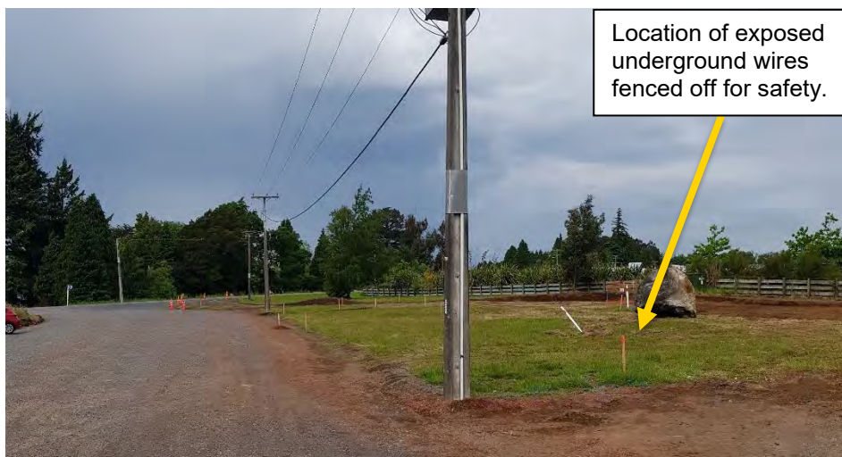
Figure 2 Fenced off Exposed Underground Wires
