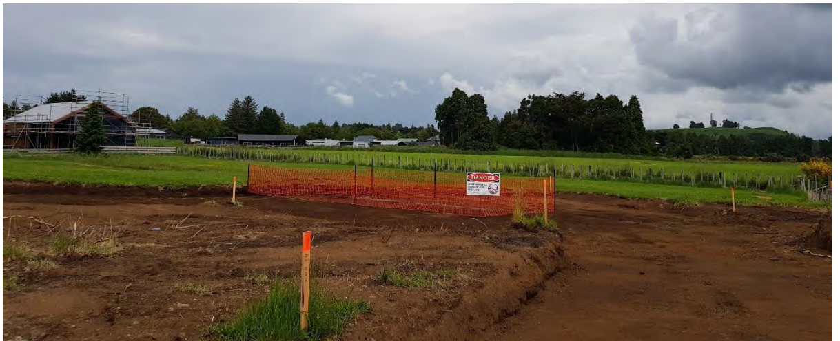
Figure 1 Isolated Sewage Field Drain
