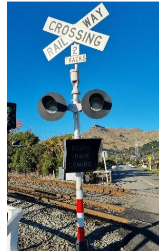
Figure 4-14: 'Second train coming' active sign
