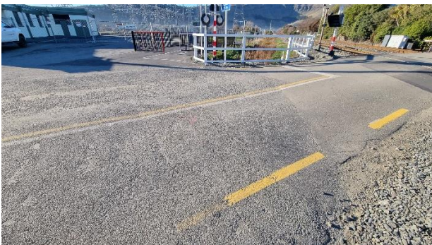
Figure 4-11: Faded line markings, no parking lines
