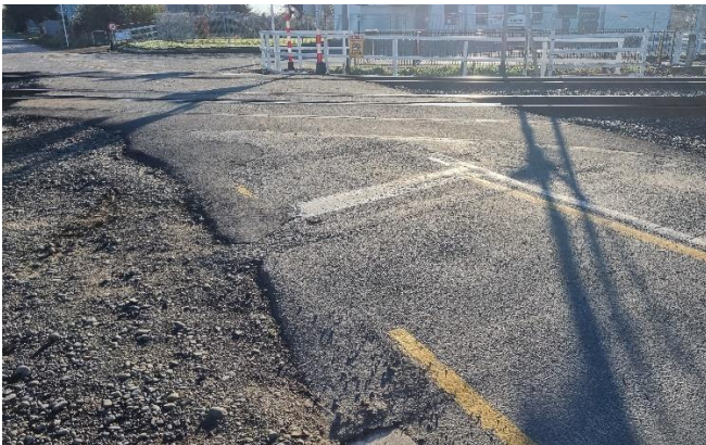
Figure 4-9: Edge break and faded line markings
