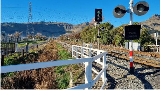
Figure 4-7: FLB with "RAILWAY" crossbuck sign and east track sightline on the northern approach
