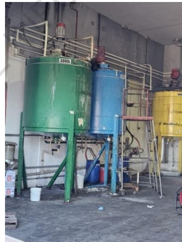
Fig1 – 9(2)(a) in right hand (blue) tank in the pair, a portable ladder/platform provides access
