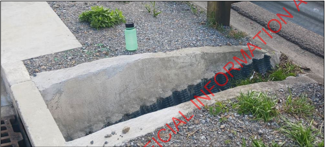
Figure 31: Example of deep, uncovered stormwater culvert adjacent to cycle path.
