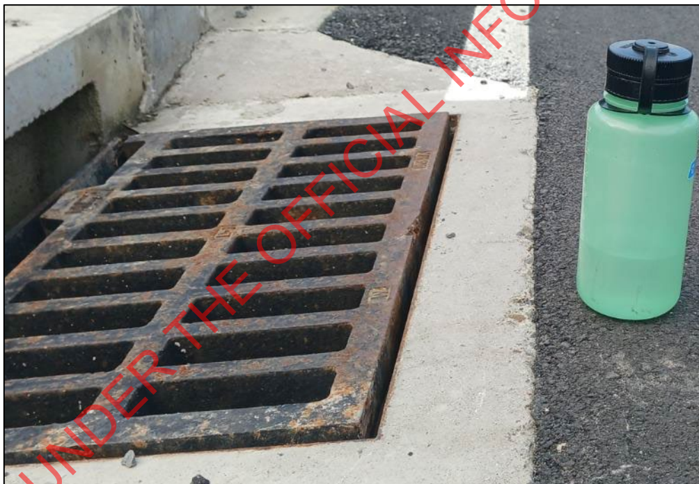
Figure 30: Example of stormwater grate protruding slightly at edge of path.
