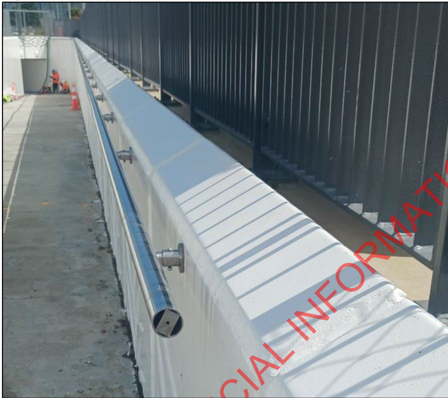
Figure 27: Service duct with no cover.
