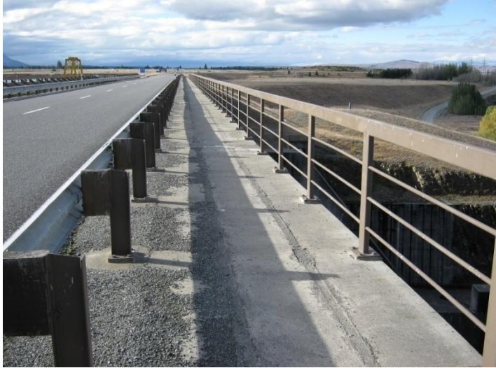
Photograph 7.2.1: Typical Hydro Access Structure
