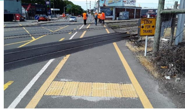
Figure 10: New asphalt panel on the siding line. Lifting of the asphalt surface is visible on the westbound lane (middle track). Note the graffiti on the look for trains signs.
