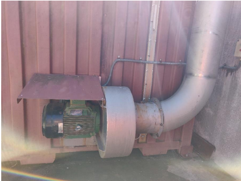
Ducting connected to the biofilter.
