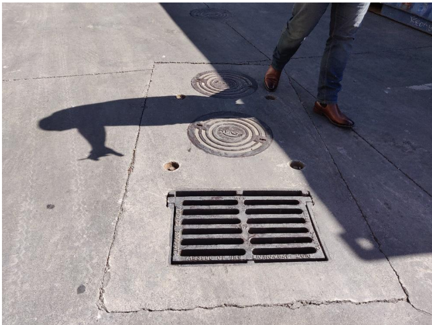
The three-tiered sump system in the driveway which is connected to trade waste.
