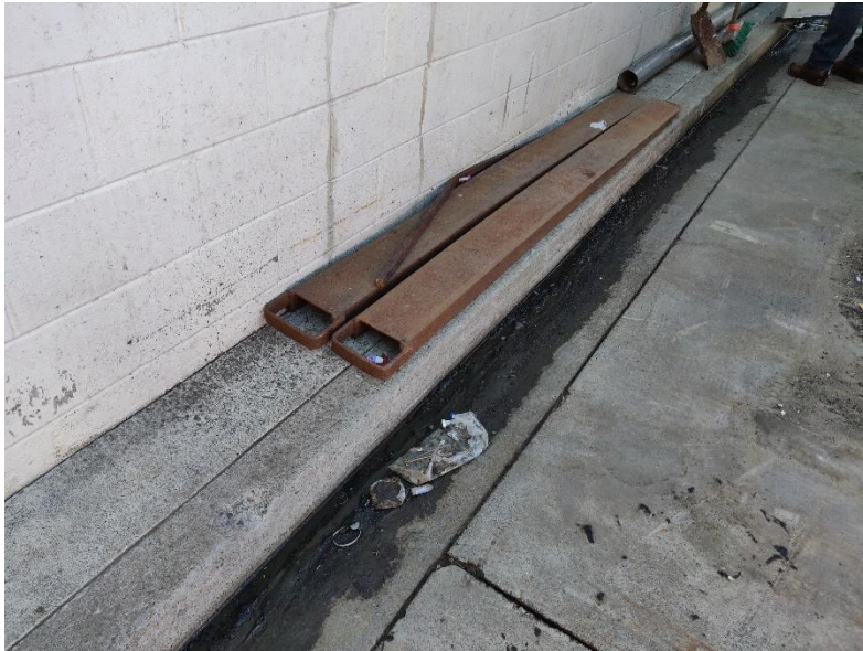
Stormwater drain along the site's northern boundary.
