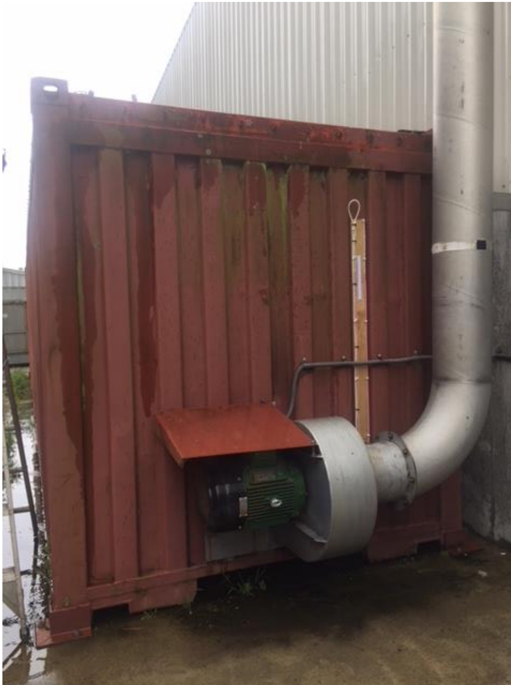
Figure 2 outside of biofilter with gauge and vent
