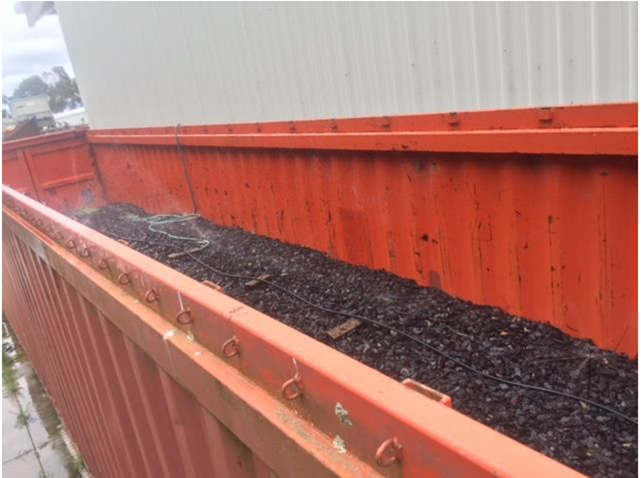
Figure 1 top of biofilter and sprinkler system
