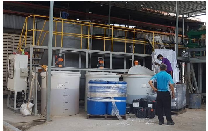
Compact water treatment unit at plastic recycling facility
