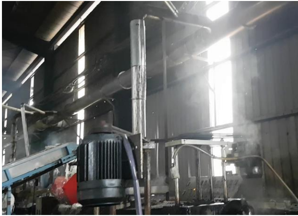
Discharge from the heating of plastic collected through ducting system
