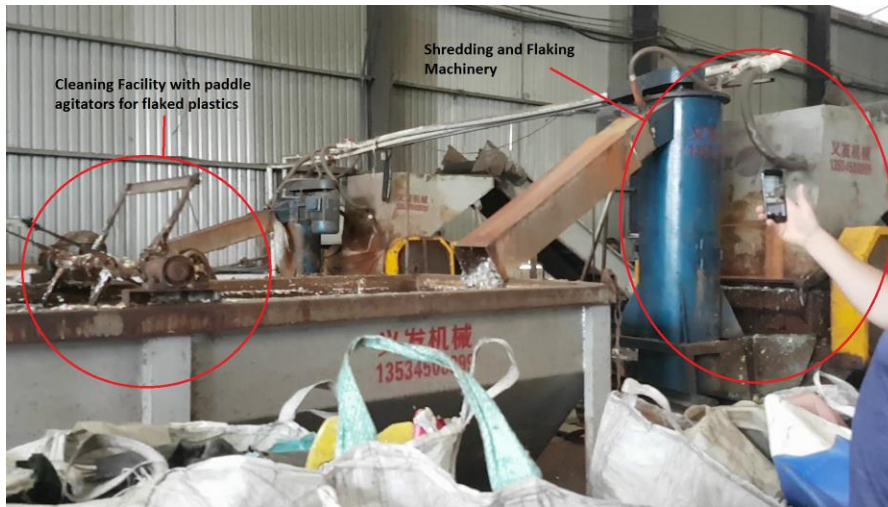
Flaking/Shredding and cleaning unit at hard plastics facility
